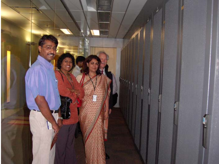
Tour of Net App's high efficiency data center with cold aisle isolation.
